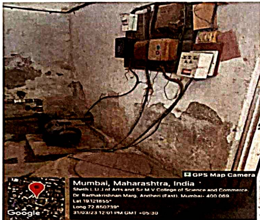
MOTOR FOR BMC WATER DISTRIBUTION TO TANKS
