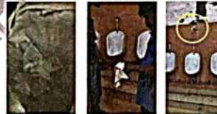
Photo 1: Comphor tablets - Polyurethi - Installed in the washroom areas
